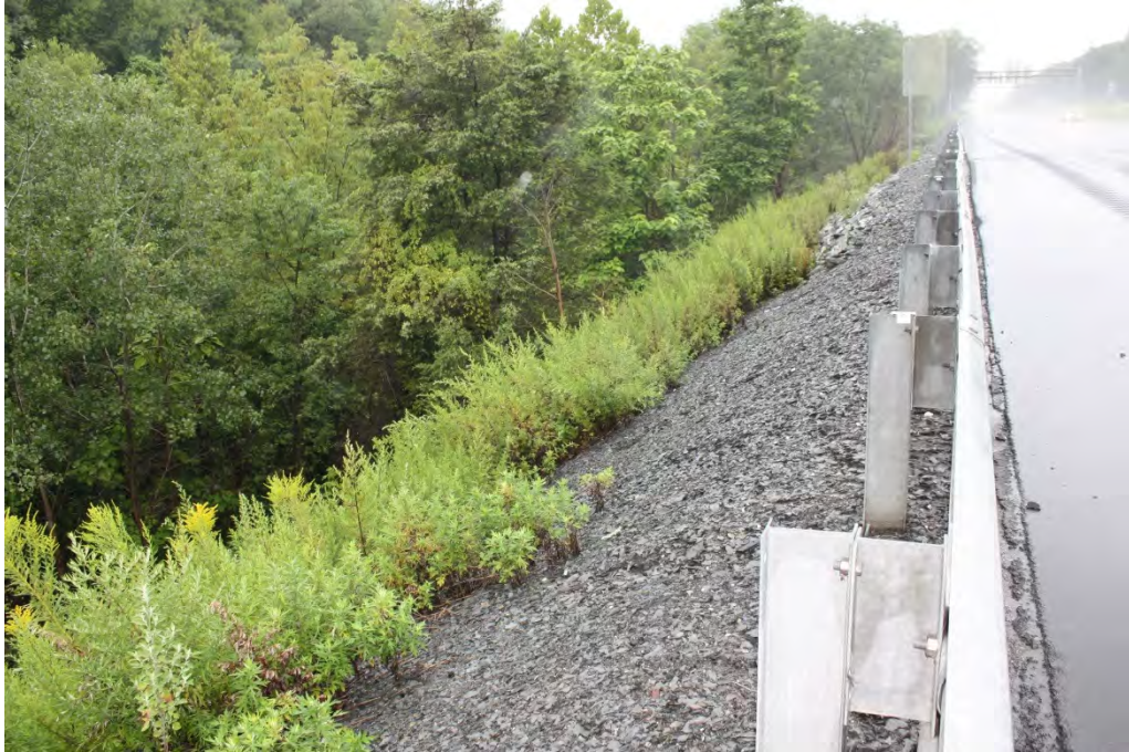
Photograph 5: General view of representative override area containing disturbance and steep slopes along the I-80 corridor. Photograph taken along eastbound I-80 between White Stone Corner Road and I-80 Exit 303, facing west.
