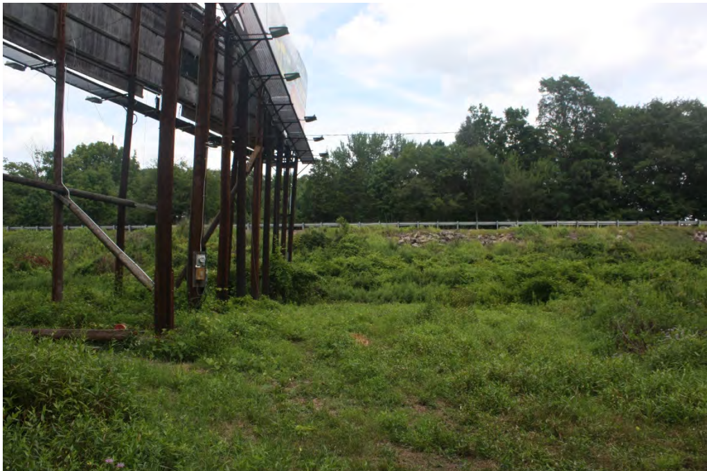
Photograph 6: General view of representative override area containing disturbance and steep slopes along the I-80 corridor, facing north. Photograph taken along eastbound I-80 west of Pocono Creek.
