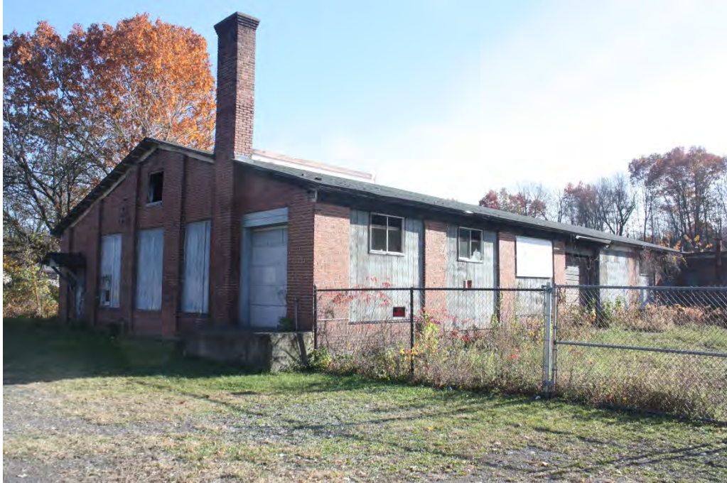
Photograph 51: General view of west and north elevations of early twentieth century Perfection Shoe Machinery Co. industrial building at 36MR0272, facing southeast.
