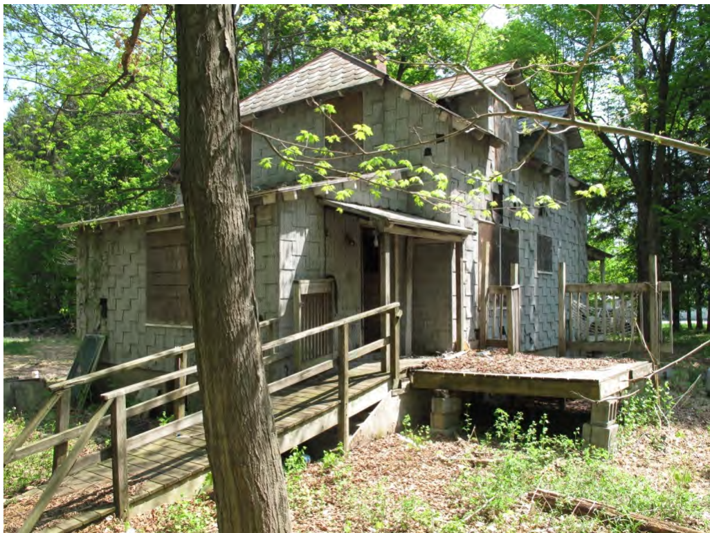
Photograph 4: View looking northeast at the west and south elevations of the Palmer House.
