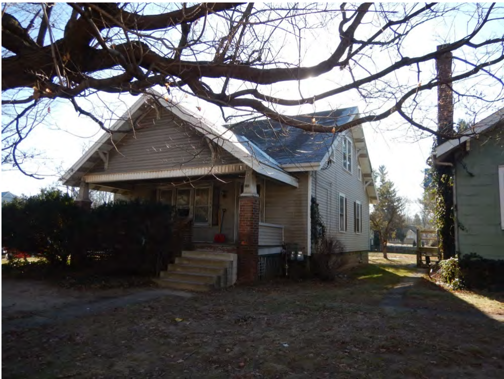
Photograph 8: View looking southeast at the north and west elevations of the house at 1817 W. Main Street.
