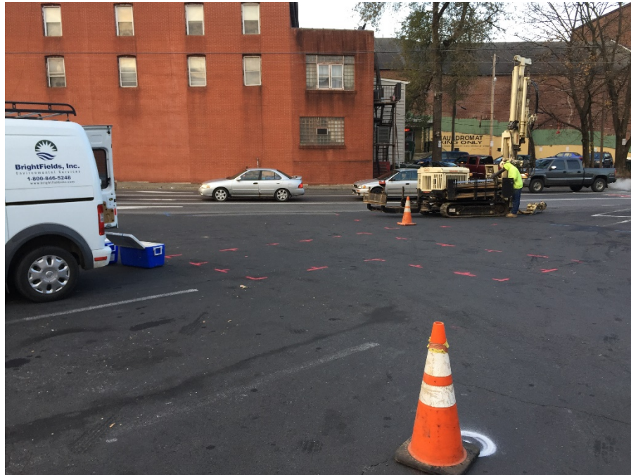
Former Gas Station site: GPR mark out visible, geoprobe rig being set up.
